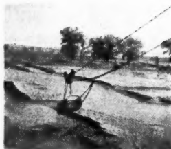
The 1 yard Sauerman Bucket coming up out of Clear Creek with a heaping load.
